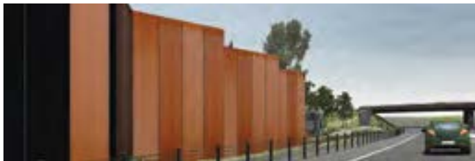
Figure 1 : Oxidised noise wall.
